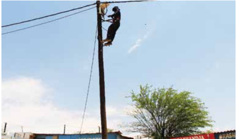
Electrician busy at work in Havana to bring electricity to the residents
